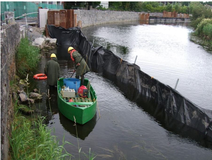
Plate 2 Fish translocation works on the Ennis Flood Scheme. In this case translocation was undertaken in advance of piling with a silt curtain suspended on a frame (Ecofact).
