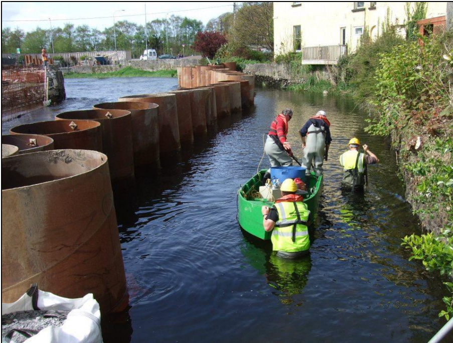
Plate 1 Fish translocation works from behind piling on the Ennis Flood Scheme. This is an example of the approach that will be taken at Enniscorthy using a boat crew and generator electrical fishing units (Ecofact).
