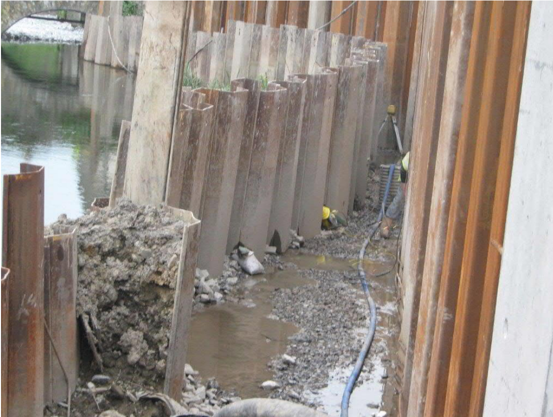
Figure 8: Example of typical steel piling impermeable barrier used within a river channel
