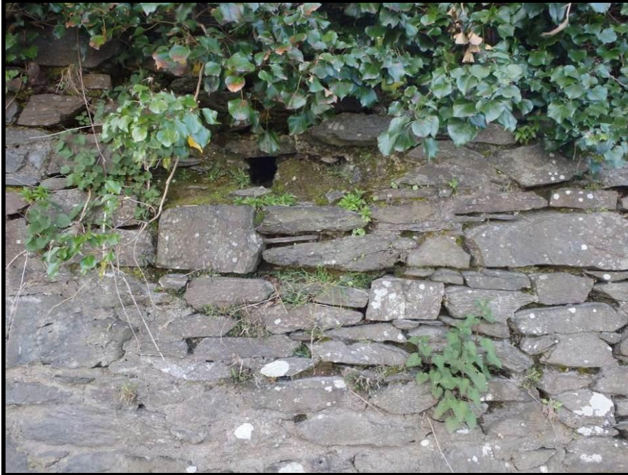
Plate 2 – Quay Walls in central and south west of the Survey Area. Note: substantial holes/crevices in walls
