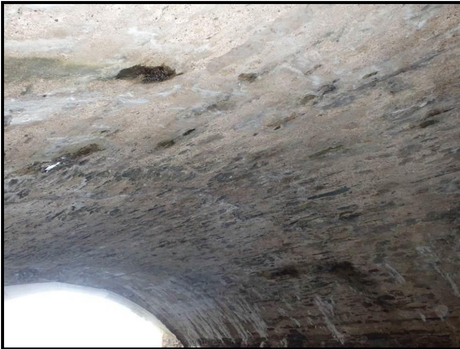
Plate 4 – A view of the typical underside of the Old Enniscorthy Bridge showing no cracks or crevices
