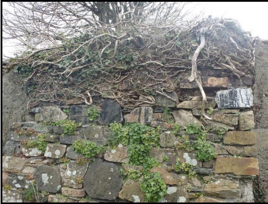
Plate 8 – The derelict building / wall on the northern floodplain
