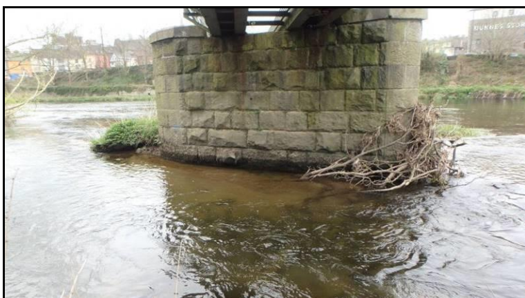
Plate 26: Many of the slower flowing areas of the River Slaney within the study area are considered suitable for the juvenile life stages of lampreys including sluggish water around pillars of bridges within the town of Enniscorthy (Site 5).
