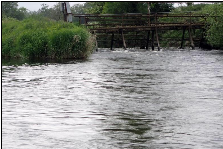
Plate 49: Tailrace screen of Clohamon hydroelectric scheme on the 26 th May 2016. Adult lampreys are likely to enter the tailrace here in significant numbers.
